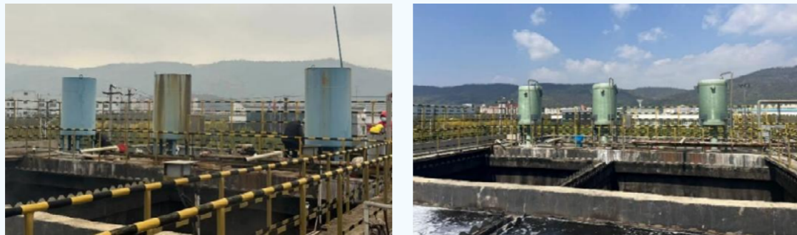
Pulse Tank for Sewage Treatment System in Qidian Industrial Zone
