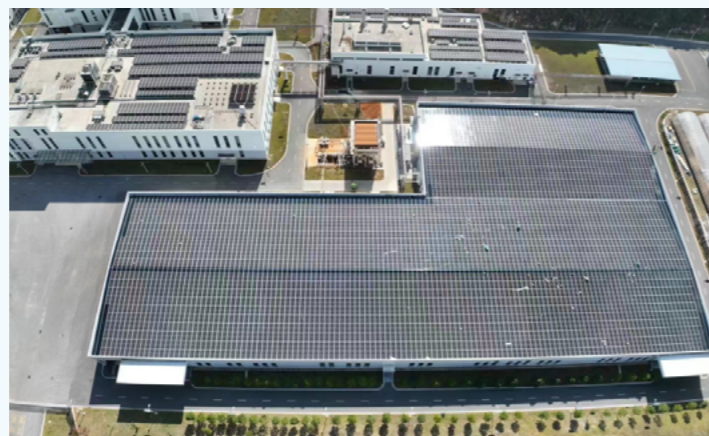
Rooftop PV Installation in Wenshan Sanqi Industrial Park
