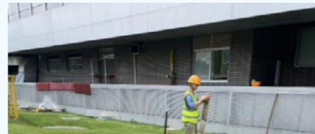
Upgrade and Modification of Electrical Fire Monitoring System
